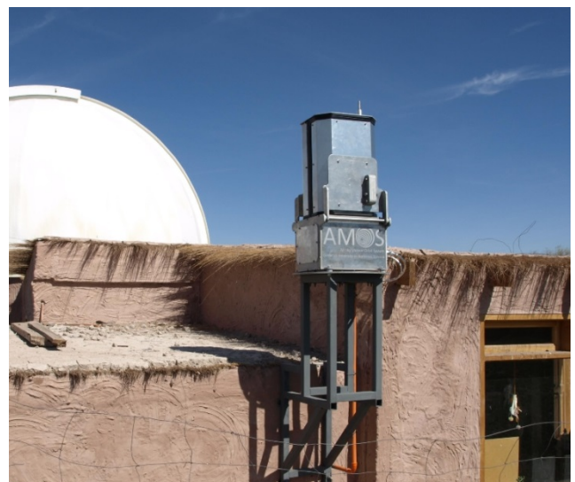
Figure 5 – Installed AMOS in Paniri Caur Observatory.
